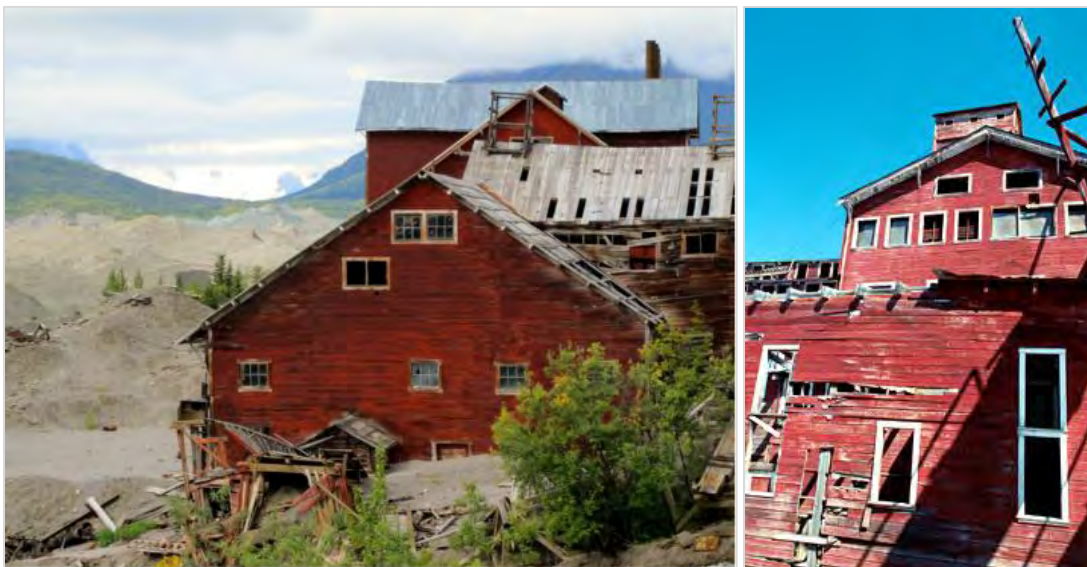
MANY OF THE BUILDINGS WITHIN THE WRANGELL-ST. ELIAS NATIONAL PARK IN ALASKA HAVE BEEN ABANDONED FOR MORE THAN 60 YEARS AND ARE CRUMBLING, DETERIORATING AND DANGEROUS. 36
