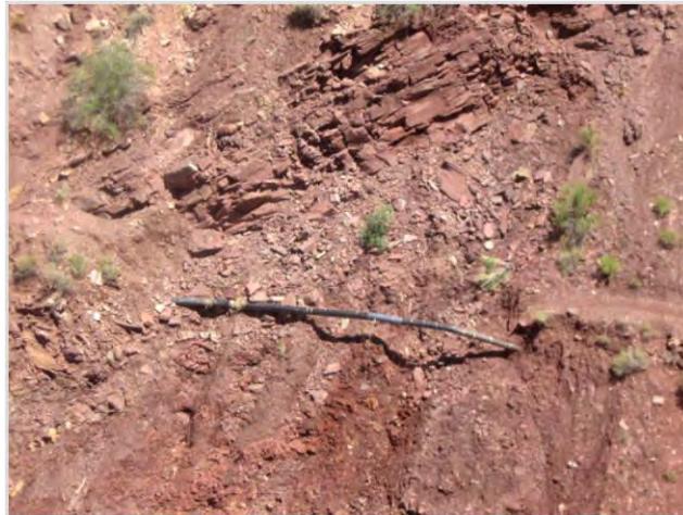
IN MAY 2012, MULTIPLE PIPELINE BREAKS CAUSED A FORTY-FIVE FOOT SECTION OF THE TRAIL TO FAIL, RENDERING CROSS-CANYON TRAVEL IMPOSSIBLE FOR HIKERS 64
