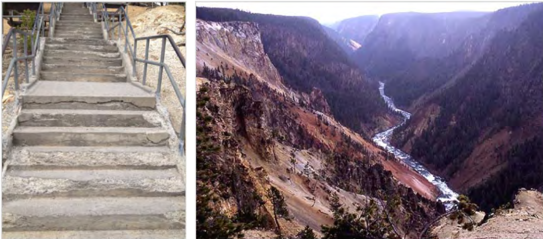
SAFETY CONCERNS POSED BY CRUMBLING STAIRS FORCED THE NATIONAL PARK SERVICE TO CLOSE THE STEPS AND POPULAR INSPIRATION POINT VIEWING PLATFORM AT THE GRAND CANYON OF YELLOWSTONE. 78
